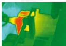
Motor: Bearing Problem
